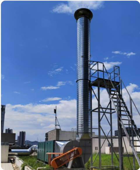
Waste Gas Disposal Facilities and Exhaust Duct
