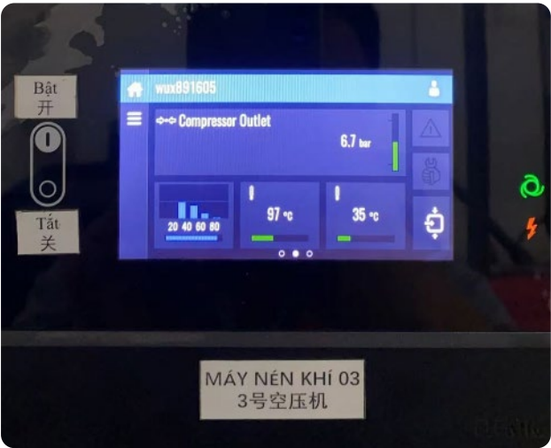
Compressor Display Screen
